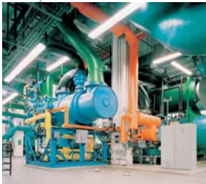
Enwave District Energy Ltd.
